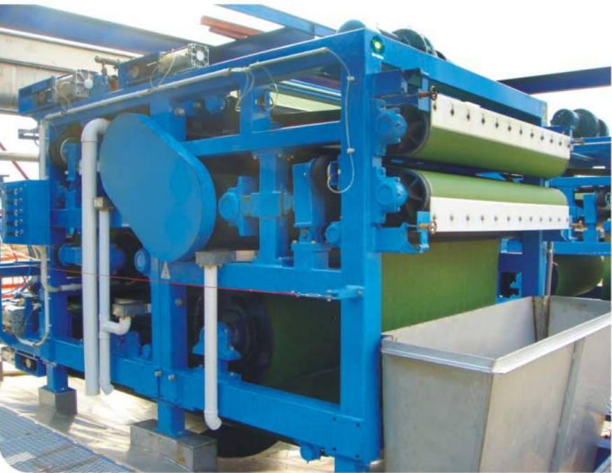
植物渣浆压榨脱水 Plant residue dewatering
